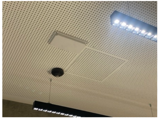
Installed AP, only antenna visible
